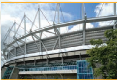
Ruskin ELF375DX louvers were installed at a 19° degree outward sloped angle facing the exterior and CD50 low leak dampers with factory actuators facing the interior. Unique issue of actuator maintenance was solved with removable blades at the bottom of each CD50 damper.
