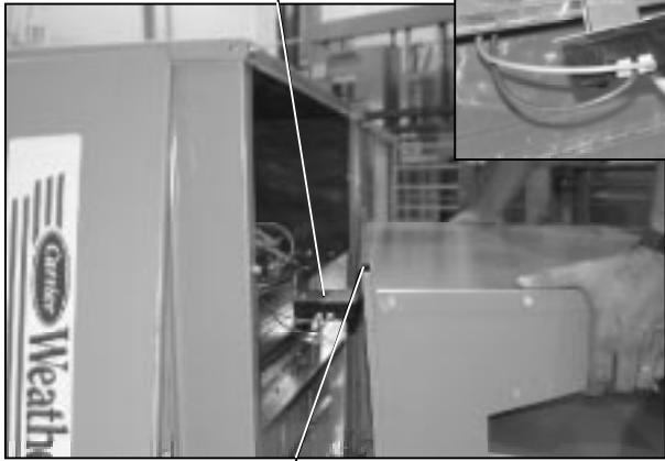
Hook over top flange of economizer
